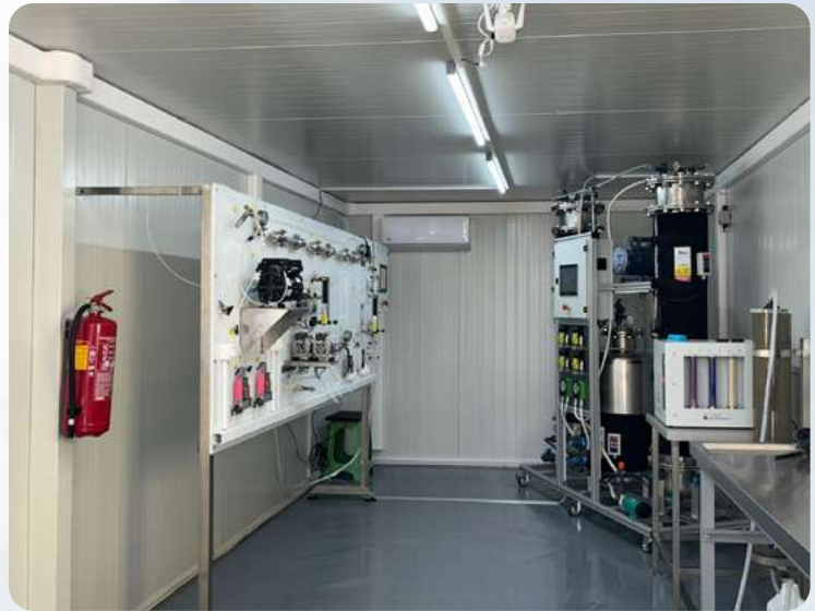
Figure 1. The mobile unit for hybrid energy storage was installed in Agios Dimitrios Plant, next to the desulfurization unit of the plant's fifth chimney.
